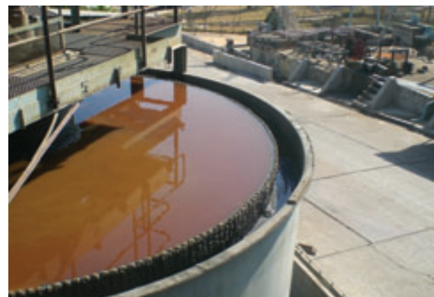
Below: The Barberton Biox plant at the Fairview operation
