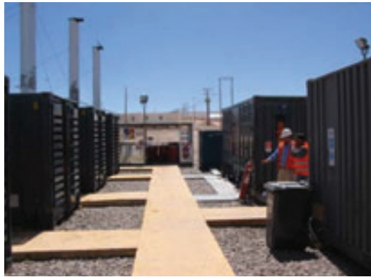
Left: Aggreko provides 5MW of temporary power to Codelco's Gaby mine in northern Chile. The 17-month contract was signed in early 2007.
