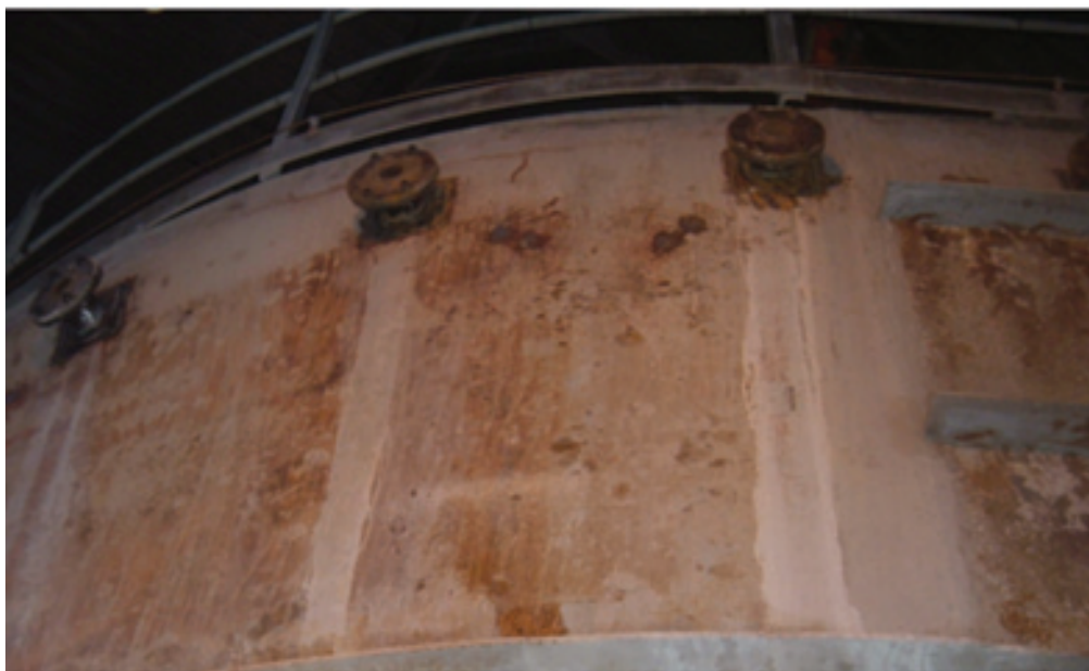
Below: Figure 2: Tubes on the outside of the cyclone through which the supports are placed.
