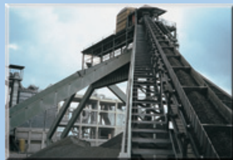
Clinker storage pan conveyor.
